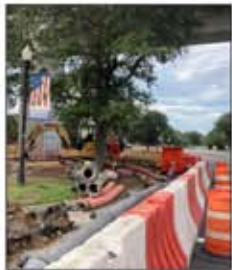
Sewer main collapses again, same cause
