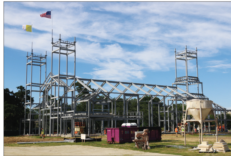
ZACH GIROUX Saint Clare of Assisi Catholic Church is slated to be complete in 2023, at nearly 22,000 square feet and an estimated cost of $22 million.
